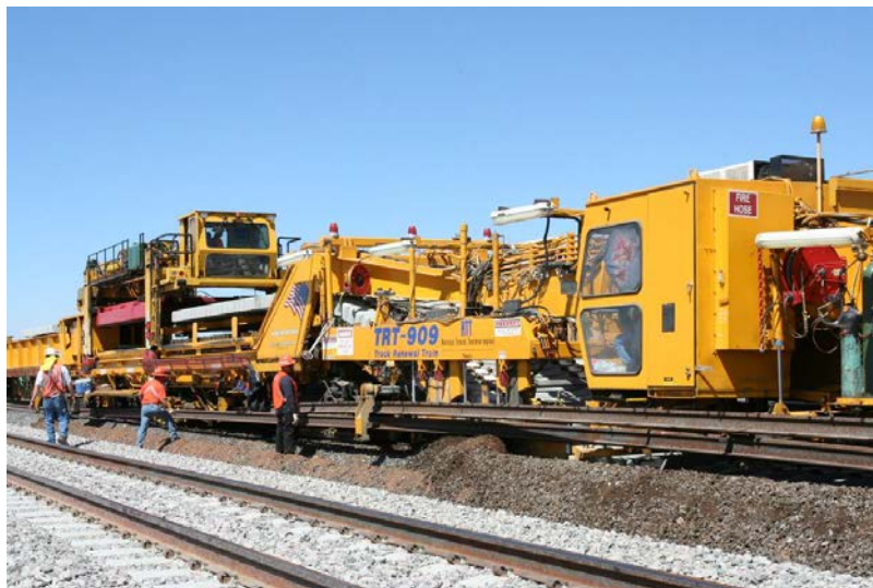
Total Track Renewal Machine Wood Sleepers to Concrete Sleepers, New Rail, Pandrol Safe-lock
